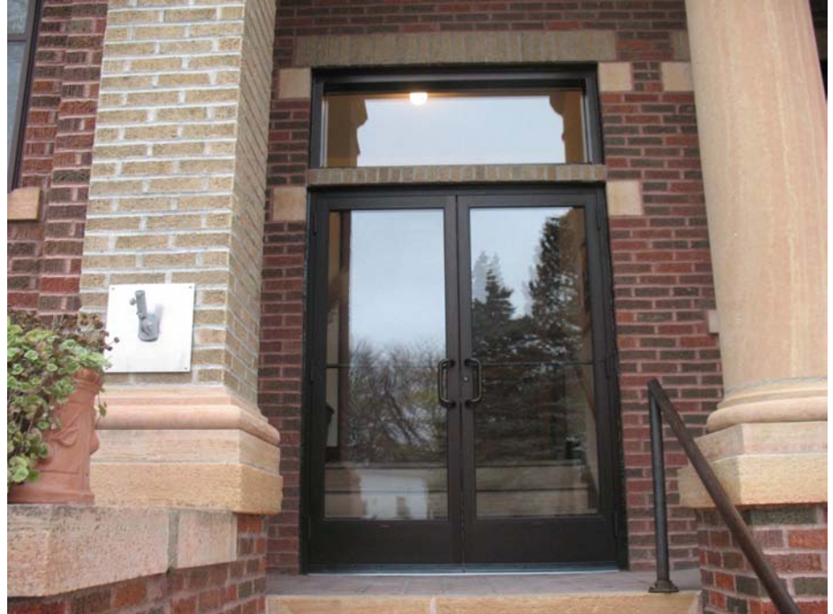
New doors installed in October made possible by a member's generous donation.
